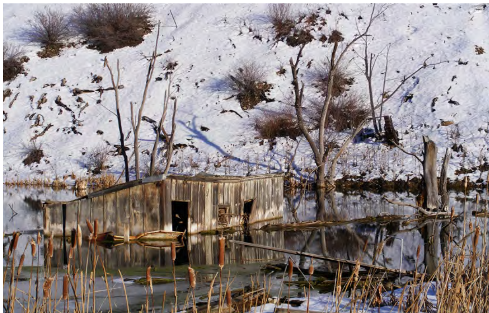
Partially Submerged Shed
